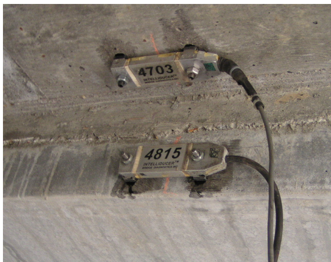
Figure 3.11. BDI strain transducers attached to concrete.
